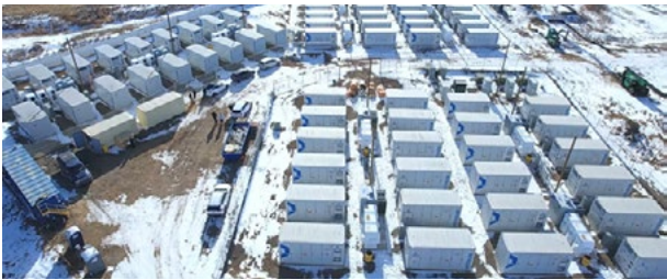
Hithium Colorado Energy Storage Project
