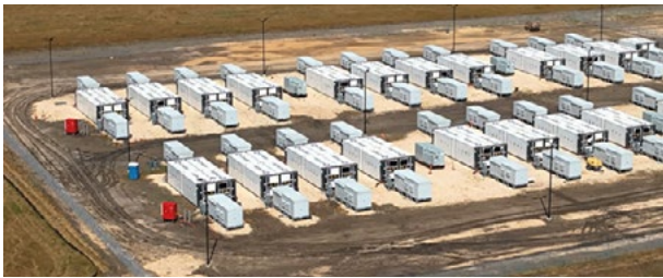
Hithium Texas Energy Storage Project
